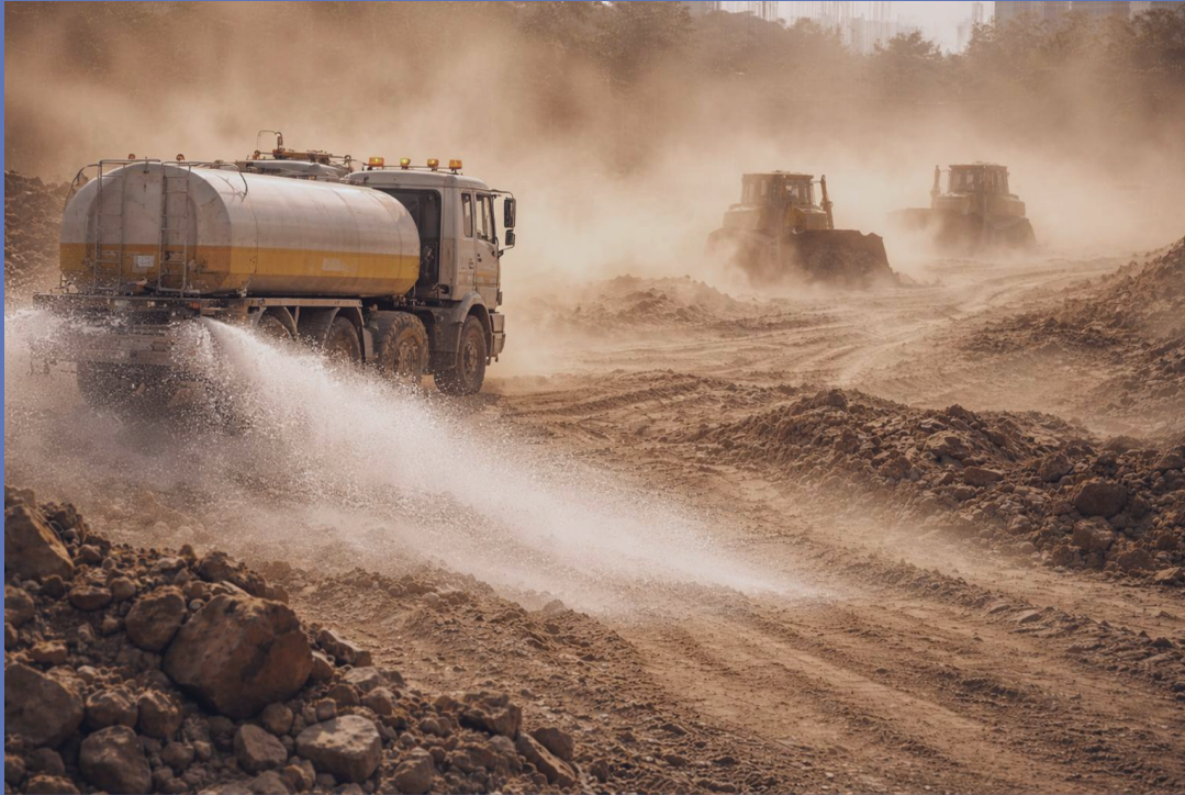
Water Application Ineffective for Dust Control
